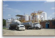
Bulk Gas Storage
