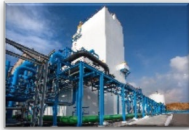
Air Separation Unit
